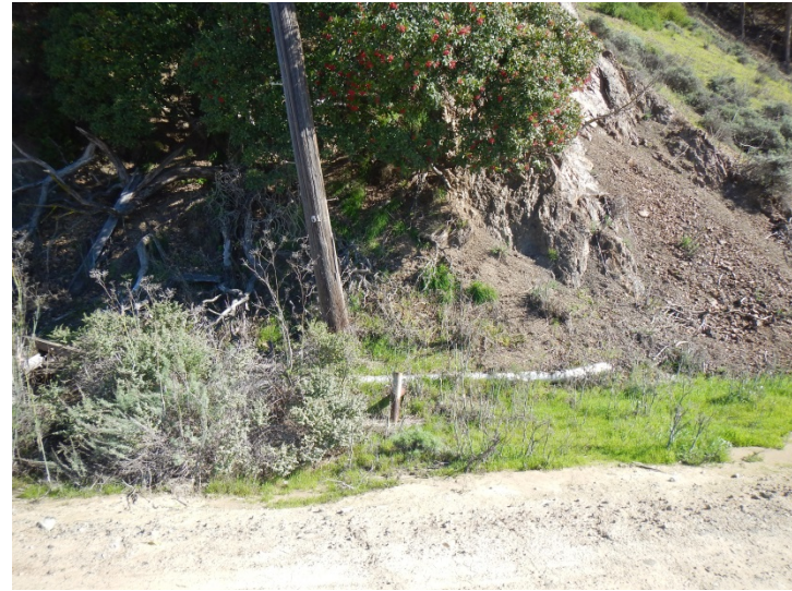
Photo 30. View facing east at surface raveling in the vicinity of OU1 Upland Cap Section TO-101 (June 18, 2014).
