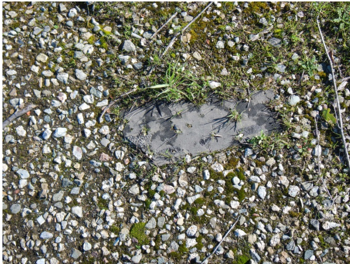
Photo 9. View of what appears to be an asbestos roofing shingle at IR Site 4 (Drum Lot 1) (February 1, 2016; Map 13)).
