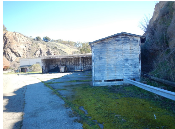
Photo 16. View facing northeast at Building 69 Pump House located in the southeastern portion of IR Site 4 (Drum Lot 1) (February 1, 2016; Plate 13).
