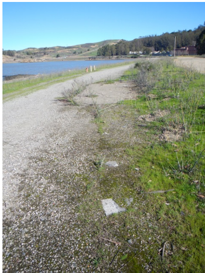
Photo 7. View facing northeast at the northwest portion of IR Site 4 (Drum Lot 1). Visible in the central portion of the photograph are what appear to be asbestos roofing shingles (February 1, 2016; Map 13).
