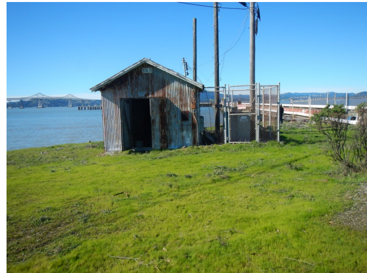
Photo 12. View facing west at Pump House located adjacent to the pier at IR Site 4 (Drum Lot 1) (February 1, 2016; Map 13 ).
