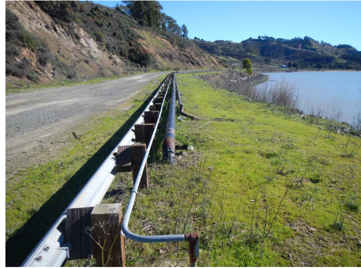
Photo 22. View facing east at former aboveground petroleum pipeline. Pipeline appears to contain asbestos coating (February 1, 2016; Map 12).
