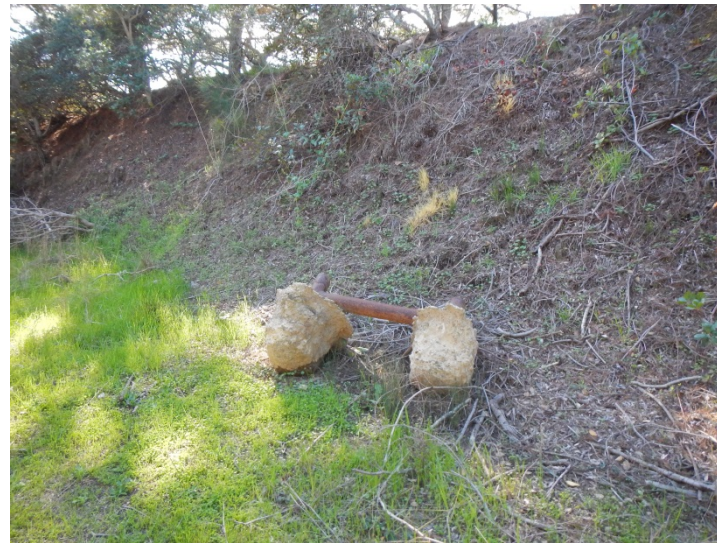
Photo 38. View of abandoned pipeline supports in the southern portion of Segment B (February 1, 2016; Map 7).
